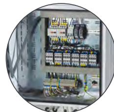
Electrical panel with protection (IP44)
